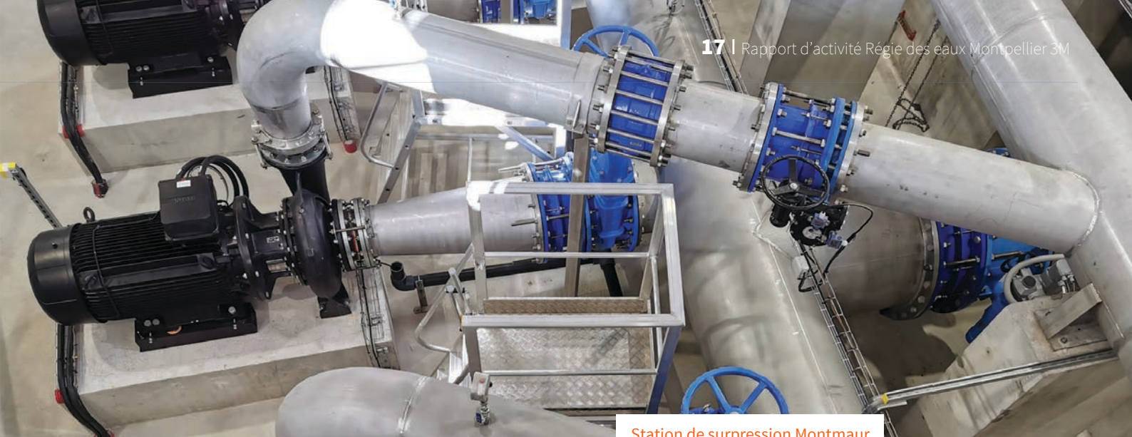
Station de surpression Montmaur
